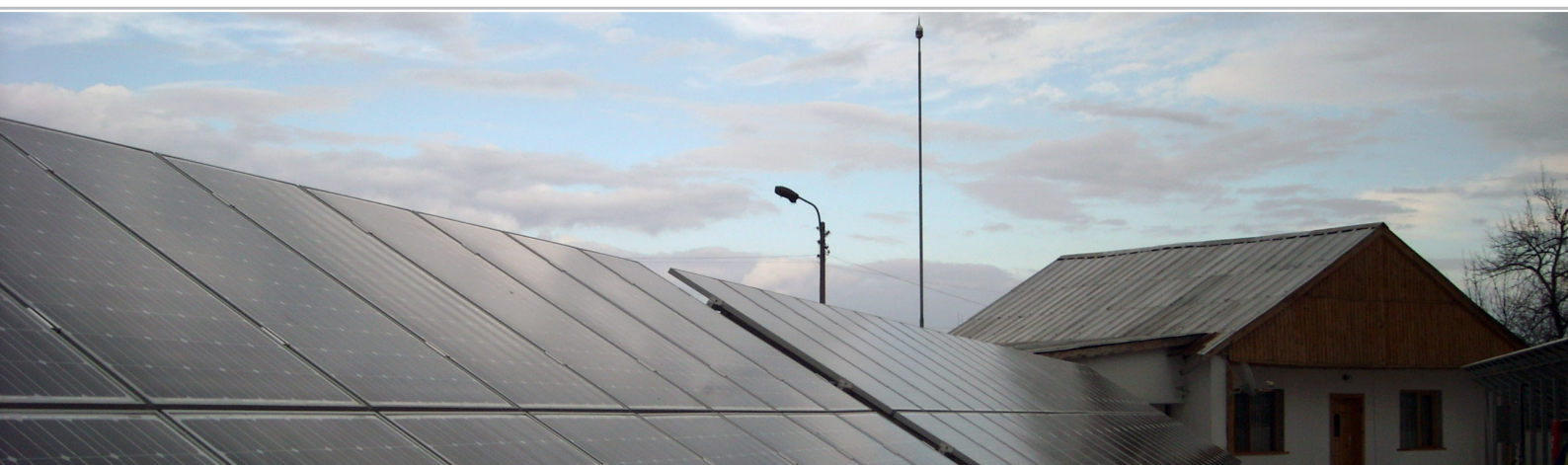
Ground solar plant
