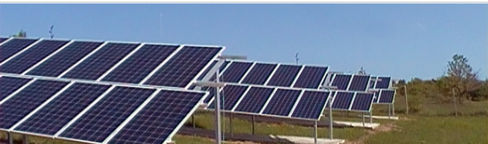
Ground mounted solar power plant
