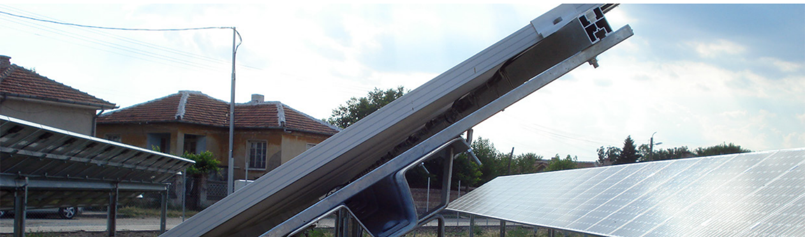
Ground mounted solar power plant
