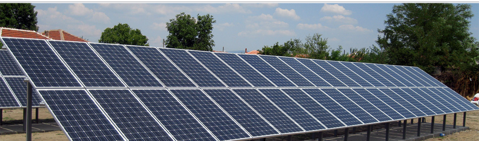
Ground mounted solar power plant
