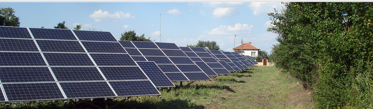
Ground mounted solar power plant
