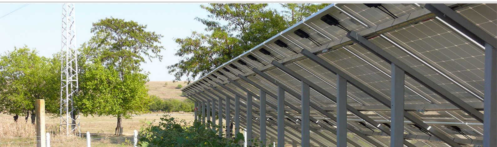
Ground mounted solar power plant
